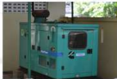
Common Area Power Backup
